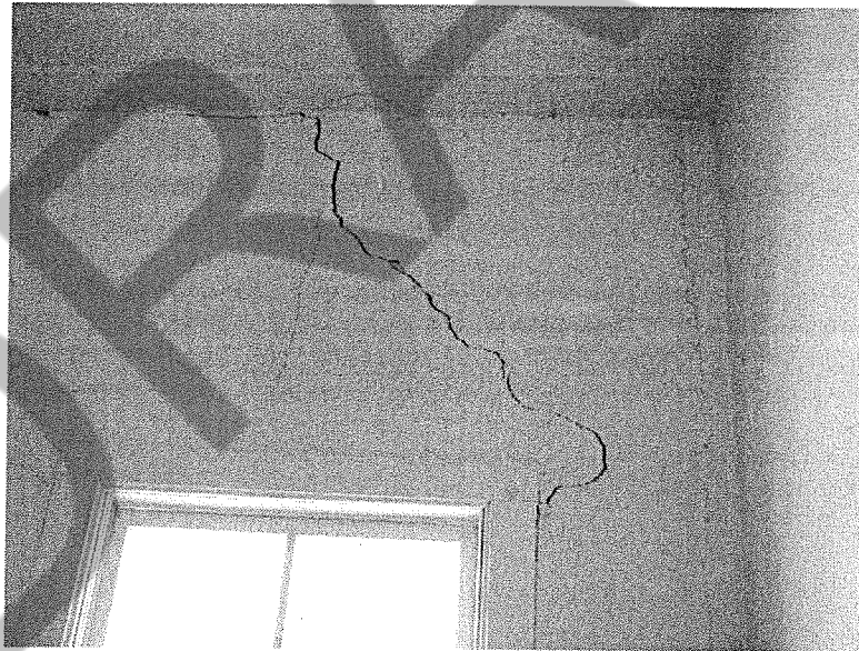
Crack in the stairwell wall. Photograph taken March 18, 2020 by J. Michael Joki, MAI, SRA
